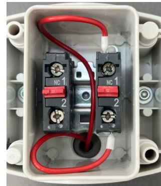
Figure 24: Cabling emergency stop
