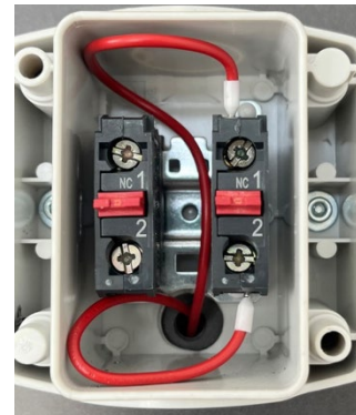
Figure 24: Cabeling emergency stop
