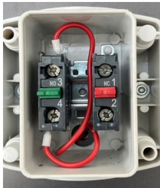
Figure 23: Cabeling key switch
